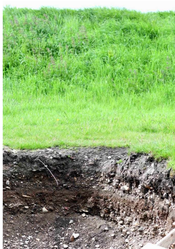
Fig. 2. Porton House crevasse splay 26 May 2021. Section immediately below seawall embankment.
